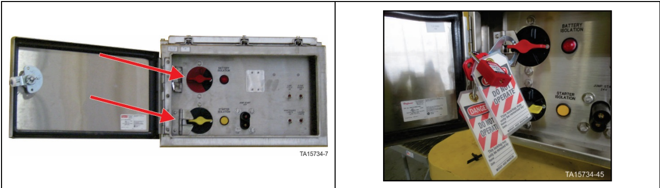
Isolation and Control switches assembly – Battery isolation switch in OFF position with locks in place
