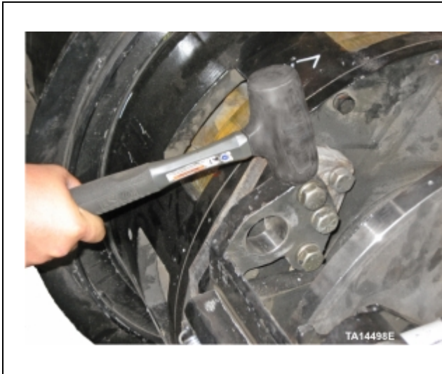
Figure 31. Tapping on torque tube to ensure it is not in a bind prior to adjustment
